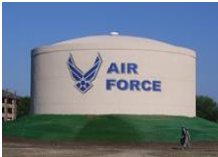
Chilled Thermal Storage
